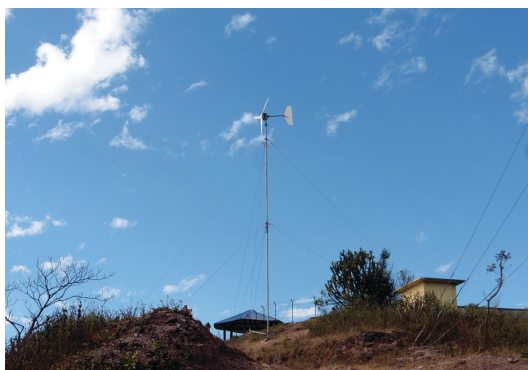
Fig: Wind Turbine installed at Palpa
