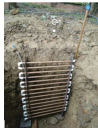
Fig: Air Water Extractor Underground Installation
